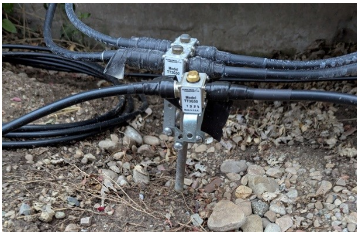
Tim's ground rod, which supports the lightning arresters, through which runs the coax for his three rooftop antennas
